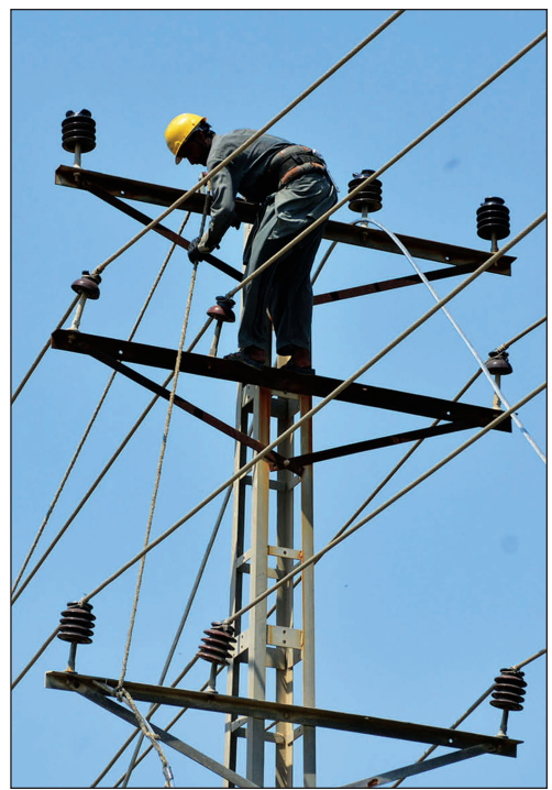
HYDERABAD: WAPDA worker busy in installed electricity cable on the electric pole at Autobahn Road. APP
